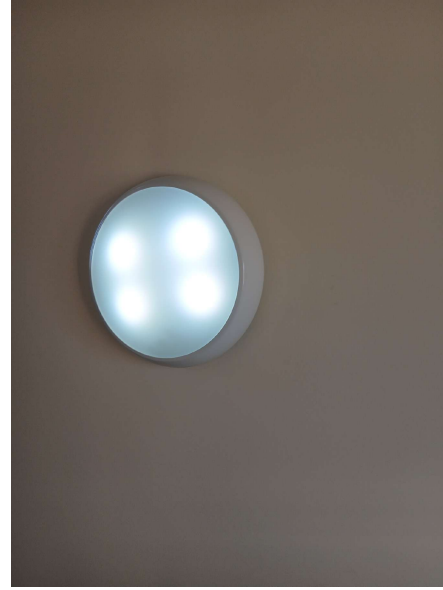
Lighting (Standard and Emergency Lights)
